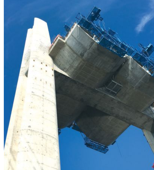
Figure 1. At the St. Croix Crossing in Oak Park Heights, Minn., a cast-in-place pier cross beam interfaces with a precast concrete segmental box-girder superstructure. In some cases, both the cast-in-place element and the precast concrete segment can satisfy their own dimensional tolerances but not match each other. All Photos: McNary Bergeron & Associates.
