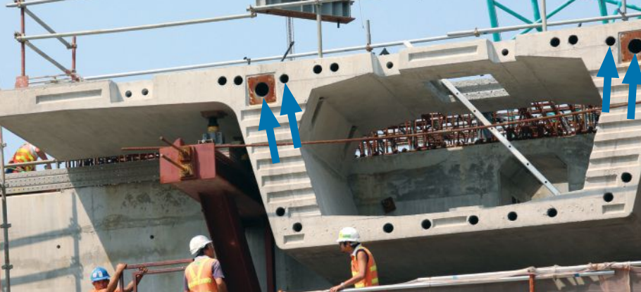
Figure 3. A precast concrete segment erected against a cast-in-place (CIP) straddle bent for the Hong Kong Mass Transit Railway's South Island Line. The precast concrete segments have been designed to sit high enough to allow top-slab tendons to pass over the CIP beam, avoiding the need to align these ducts between the CIP beam and precast segments. The deck above the top of the straddle beam is cast at the same time as the wet joint. Post-tensioning ducts near the top of the web (indicated with arrows) have been detailed slightly lower than other ducts in the top flange to accommodate reinforcing bar bend tolerances in the stirrups (see Fig. 5).
