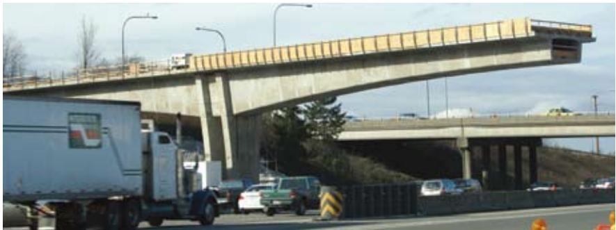
The construction system allowed the guideway to be built over I-5 with little disruption to traffic. Photo: PCL.
