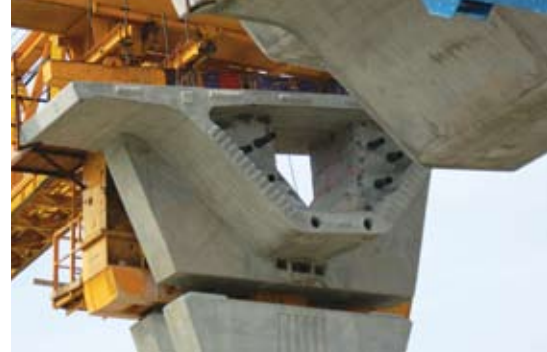
A precast pier segment is lowered into place by the overhead gantry. Photo: IBT.
