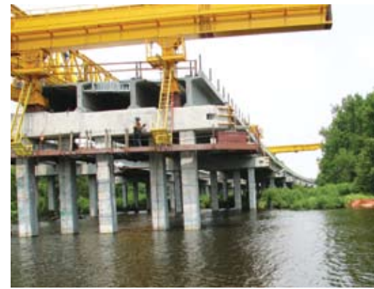
On typical spans, the gantry drives nine piles, then sets the precast concrete caps in three pieces on the piles. The caps are then post-tensioned and infill concrete placed.
