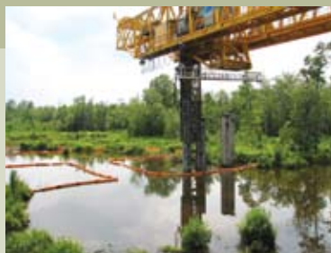
The innovative top-down construction method results in minimal disturbance to the wetlands during the construction operation. The only permanent impact is the actual pile footprint.
