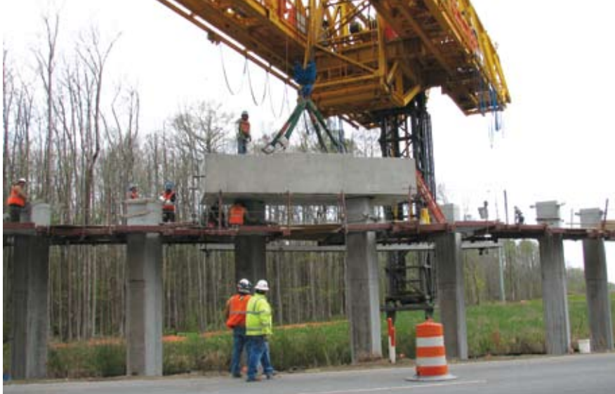
The gantry system is used to attach pile caps in three pieces to the precast concrete piles.
