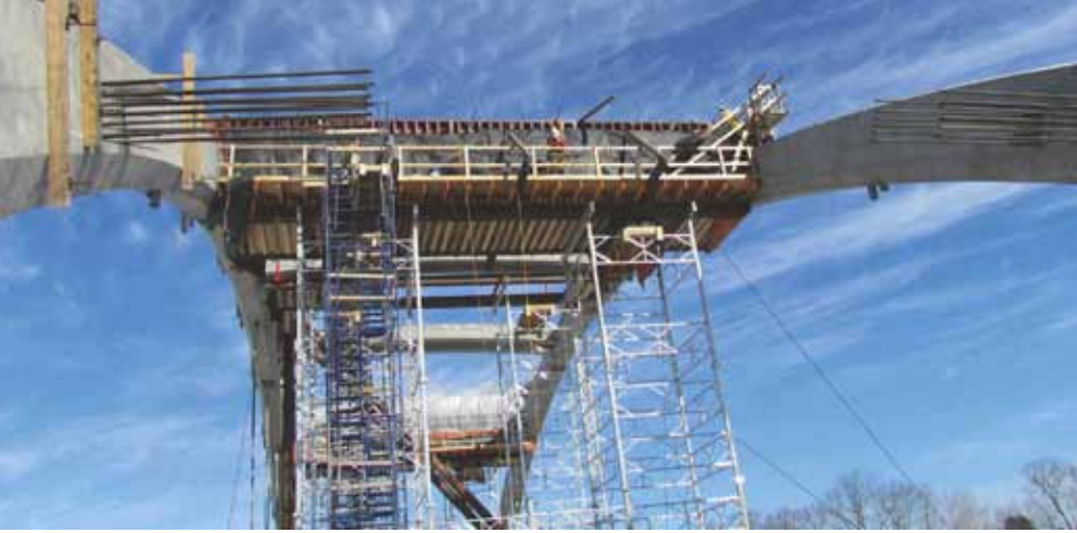
Formwork and reinforcement are nearly complete for transverse braces No. 2 and 5. Falsework and forms for transverse braces No. 3 and 4 have been removed. There are a total of six braces. Photo: Kleinfelder.
