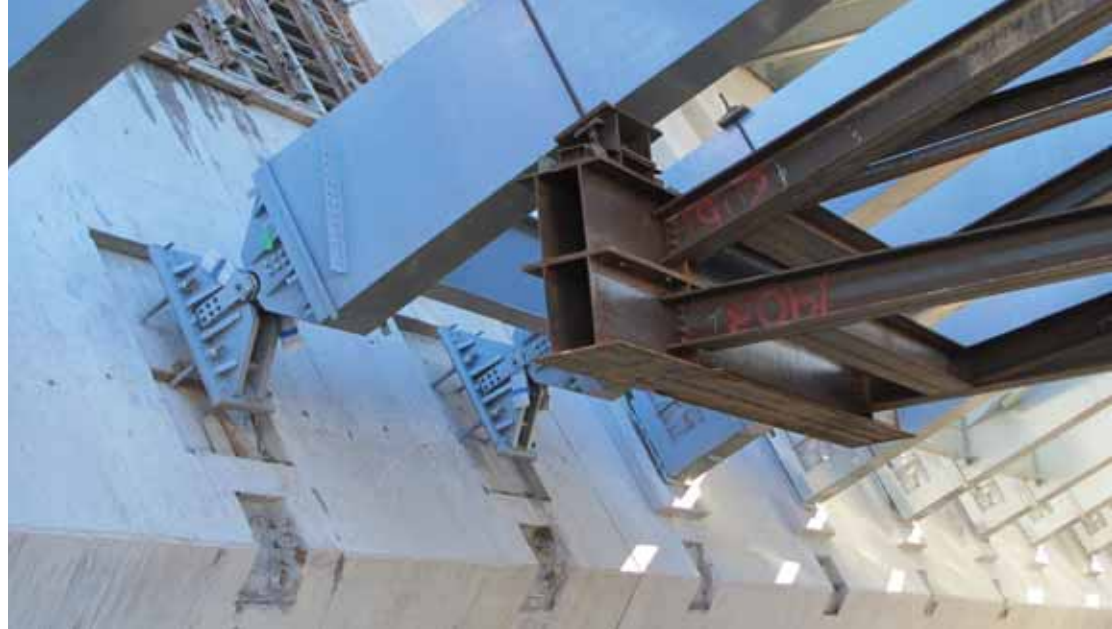
Arch ribs are suspended into place at their final destination, while bearings have been projected forward into theoretical position just before placement of concrete at the plinths.
